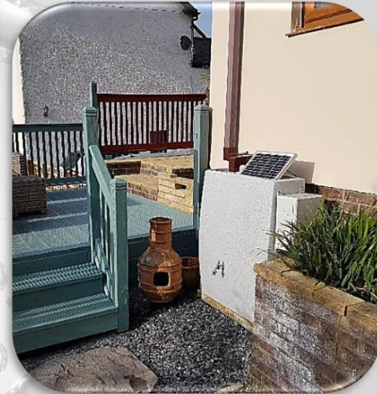
Smart Tanks can be blended in with the surroundings to provide useful water, great attenuation whilst being cost-effective and aesthetic.
